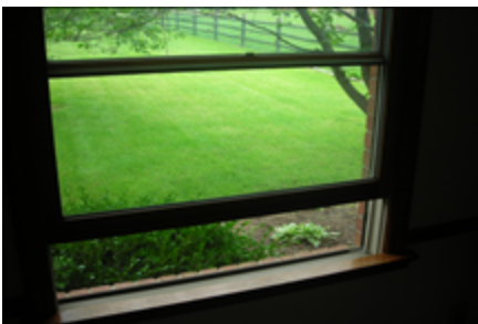
Double panel windows installed in 1999
