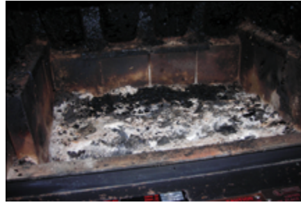
Clean and service fireplace
