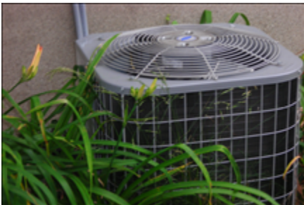
Trim vegetation away from unit
