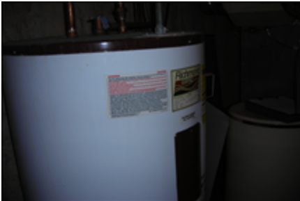
1989 rusty hot water heater
