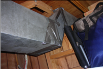
Duct tape used to seal gaps in duct.
