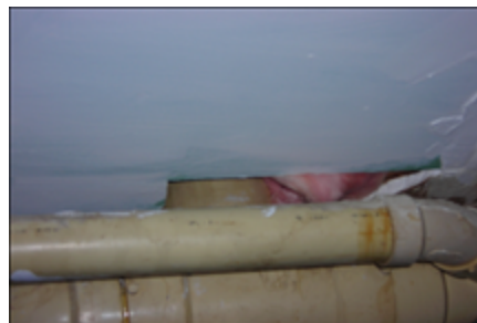
Insulation near plumbing penetration
