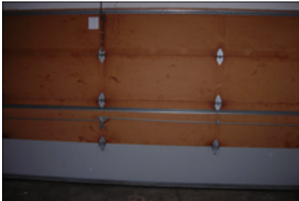
recommend insulated garage door
