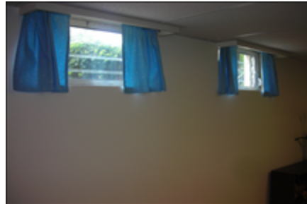
basement windows not energy efficient
