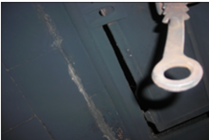
Repair defective damper
